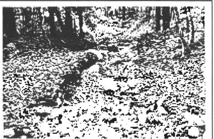
This severely eroded logging road was constructed on a moderately steep terrain. No provision was made to divert runoff from the road surface. As a result, runoff remained on the road, which over time have eroded to a depth of over two feet in some places. Material from the road washed into streams and carved additional erosion below the site.
